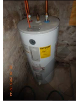
electric water heater in basement under steps to 2nd floor
