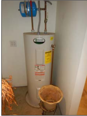
electric heater at foot of basement steps
