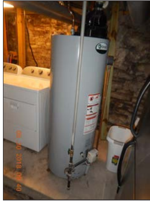
gas water heater at basement laundry
